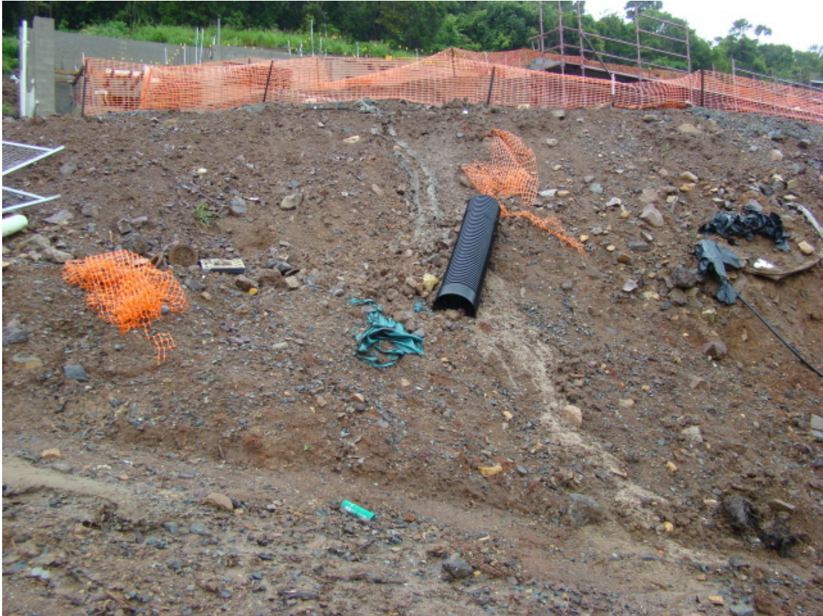
Failures of erosion management on Airlie Beach hillside, previously rainforest and Proserpine Rock Wallaby habitat.
